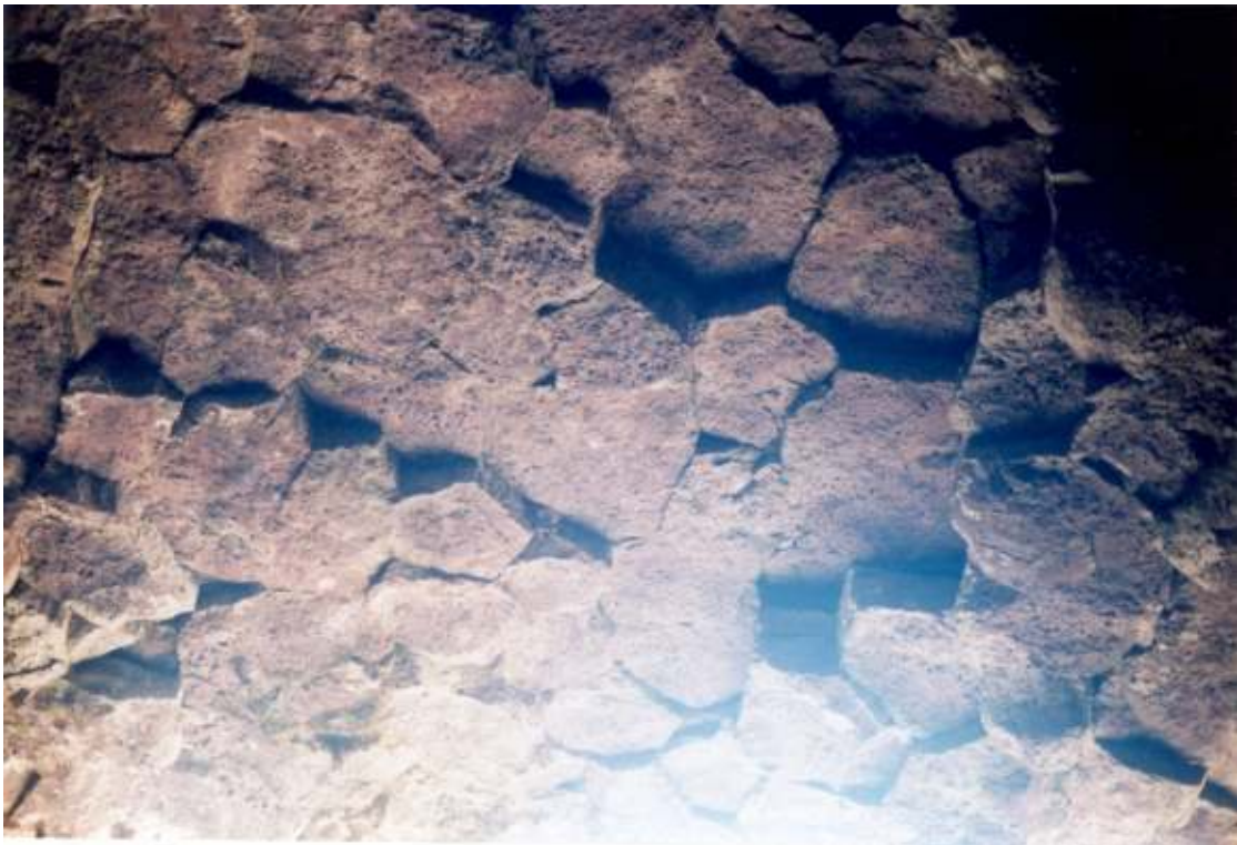
View of the ceiling in the upper level of Lava Plug Pit, with lining peeled off and revealing cross sections of columnar basalt. 6-6-06
